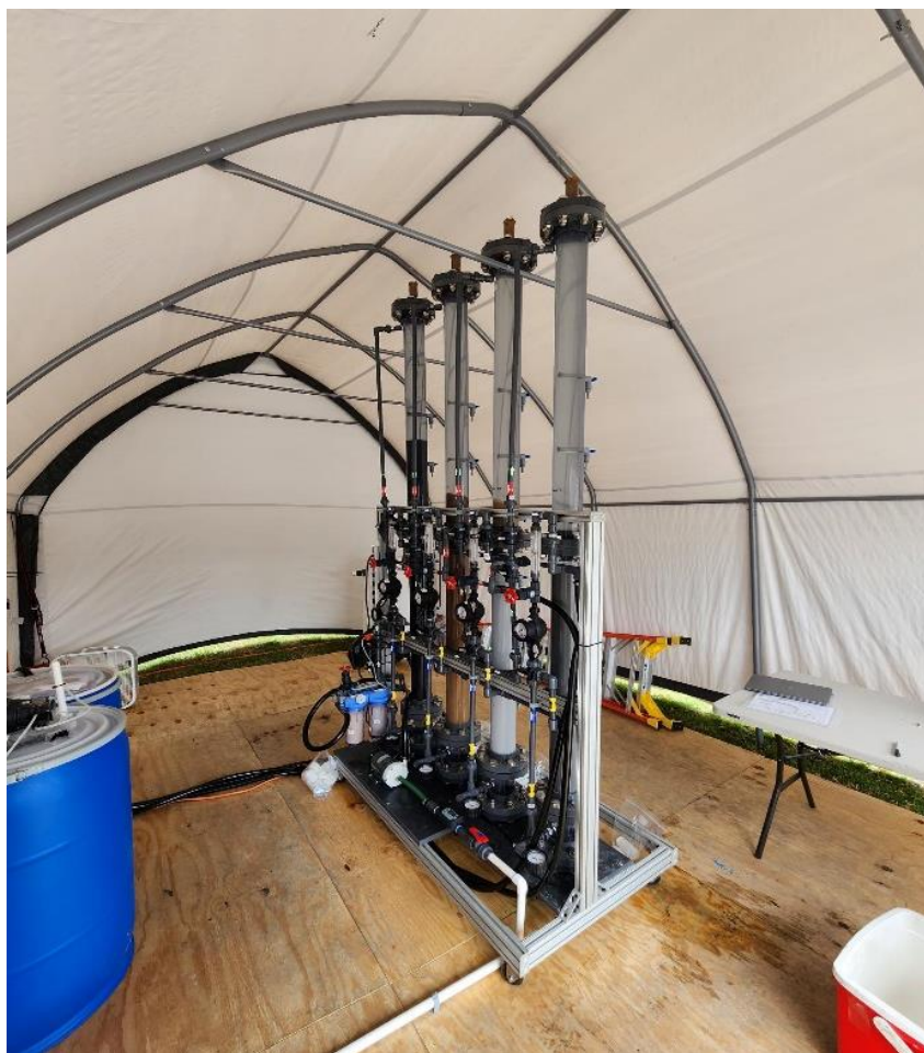
Figure 3-5: City of Margate Ion Exchange Pilot Skid
