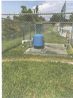
Existing Irrigation Pump
