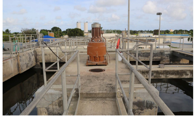
Replacement of surface aerators with IFAS technology will unlock East WWTP treatment potential.
